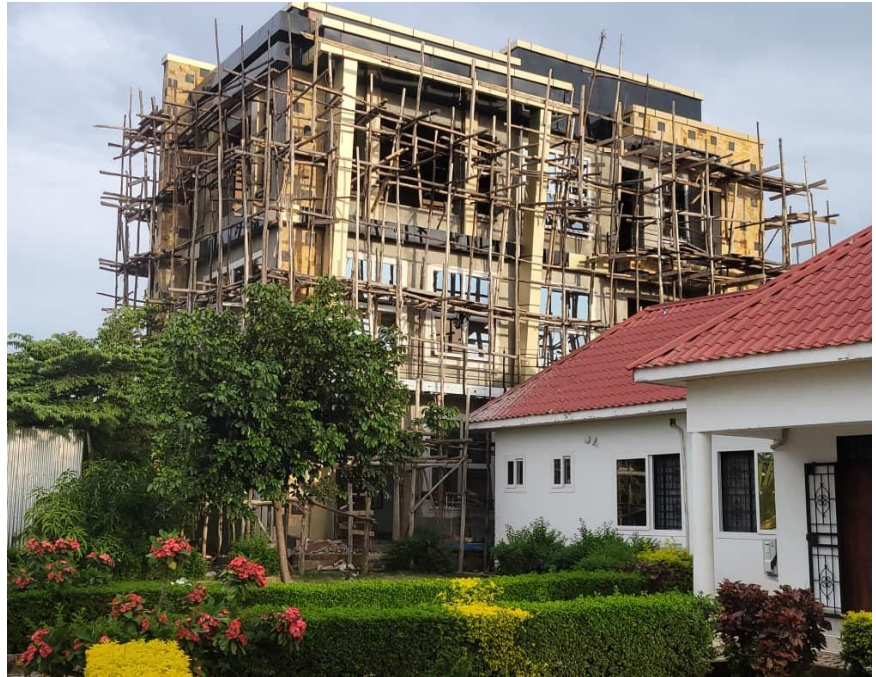
A new look of the TMA building on final touches at Itega, Dodoma
